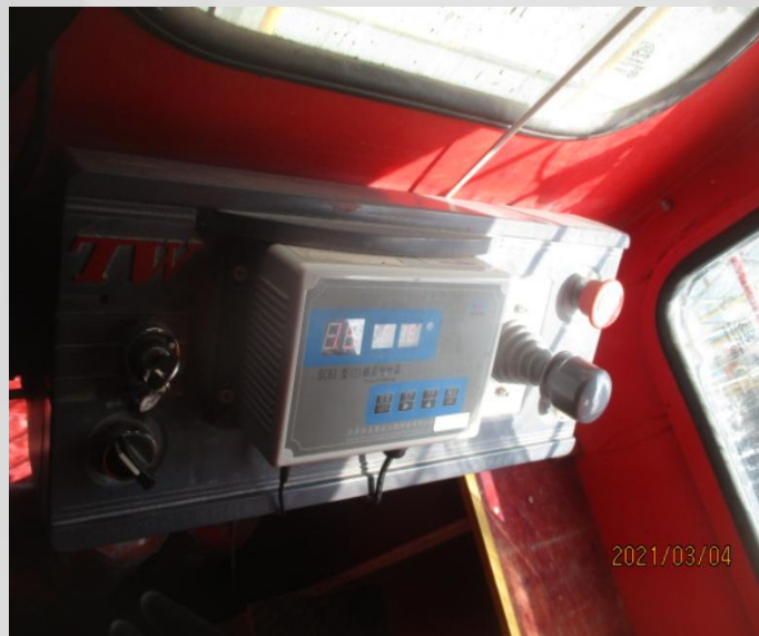
吊笼内紧急开关调试失效
